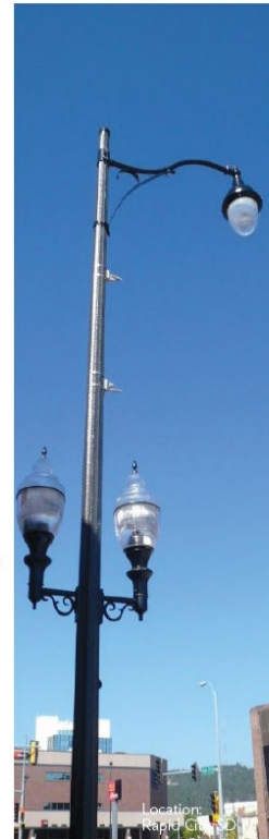
Figure 223: Decorative Light Fixture
