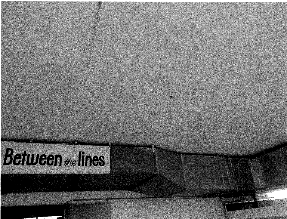
Figure 8 – Parkade Ramp – Underside Blue level slab above entrance ticket gate. Signs of potential corrosion with brown discoloration.
