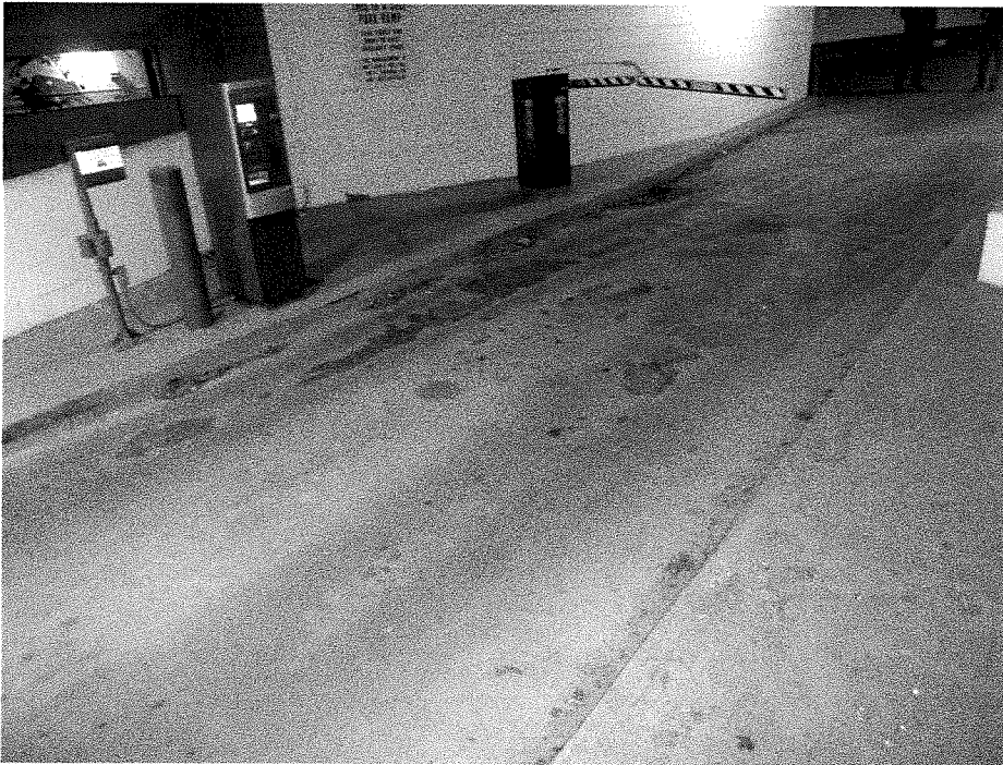
Figure 2: Parkade Ramp Entrance – Ticket machine gate. Traffic coating is worn through along wheel tracks all along the ramp entrance.
