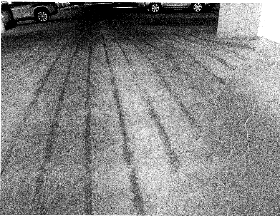
Figure 10 – Parkade – Green Level – (Photo from 2022) Recent epoxied rebar repairs near exit to spiral. Required next step is protection of these repairs with traffic coating.
