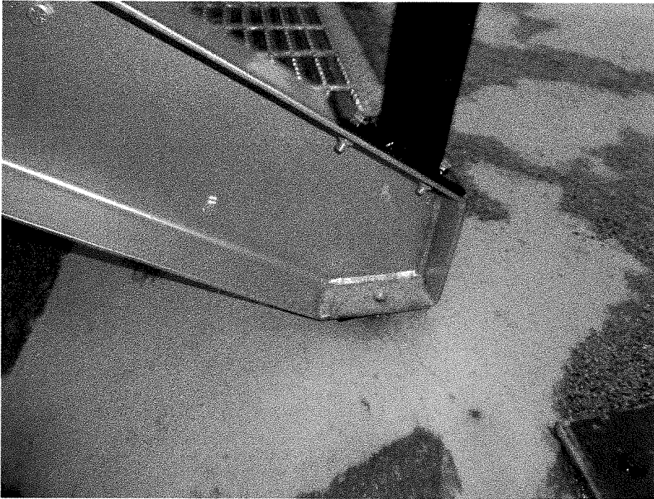
Figure 13 : Parkade – Roof Level - New exterior roof stair showing steel corrosion at the base of the stair channel. This is typical at the base of both stair channels.
