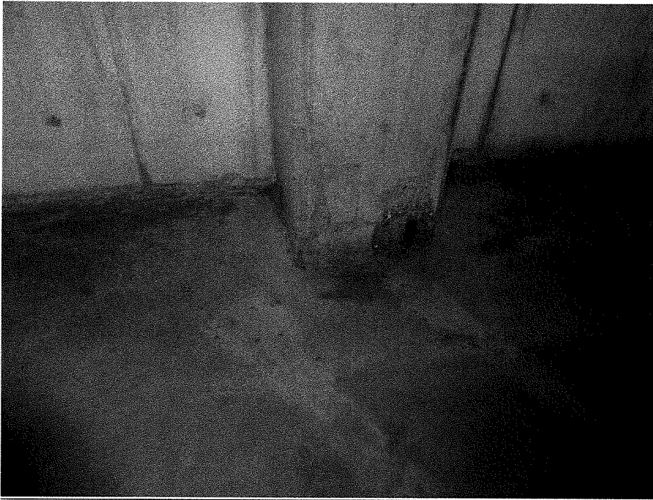
Figure 11: Parkade – Red Level – Spalling at corner of column
