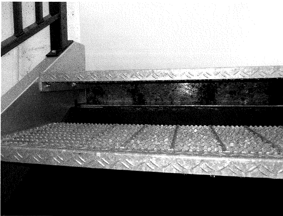
Figure 12: Parkade – Roof Level - New exterior roof stair showing steel corrosion atop the existing concrete at the top of the stair.
