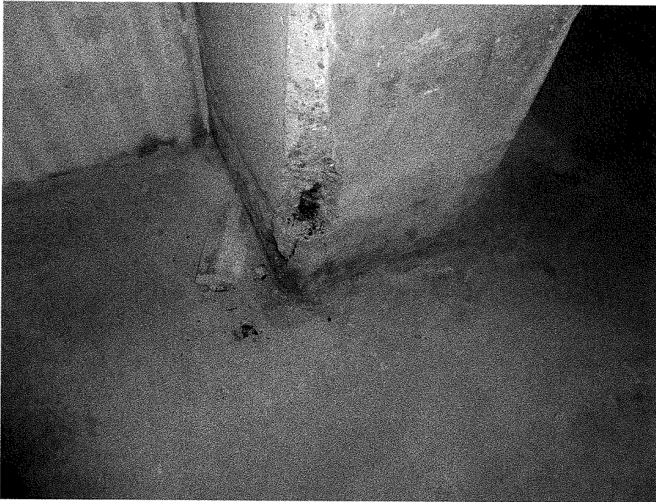
Figure 9 – Parkade Ramp – Green Level column at south side of the ramp. Base of multiple columns show signs of rebar corrosion and concrete spalling due to consistent exposure to moisture along south wall.
