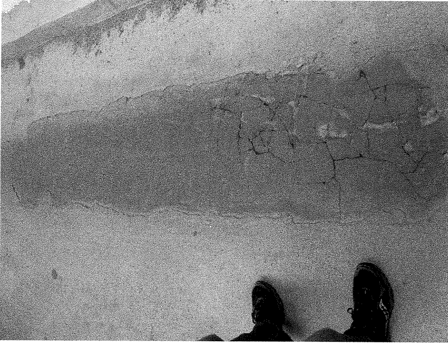
Figure 1: Parkade Ramp Entrance– Damaged traffic coating was cut away, revealing concrete delamination in prior patch. This correlates to moisture infiltration in the mechanical room below.
