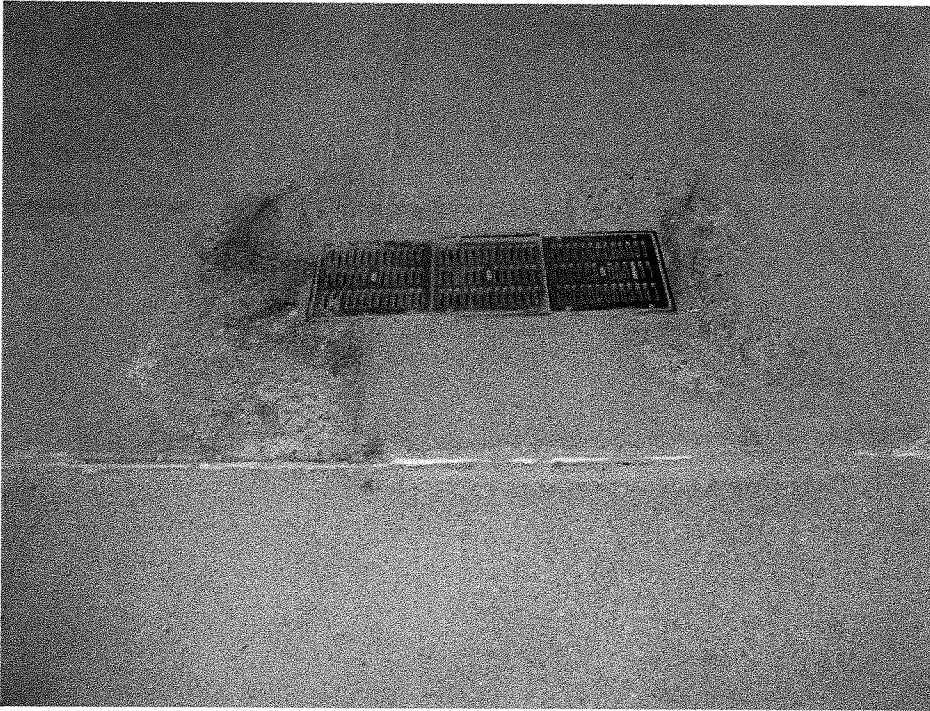
Figure 19 : 3 rd Street Ramp– Typical slab spalling around drain grate at west entrance. Typical at two entrance grates.
