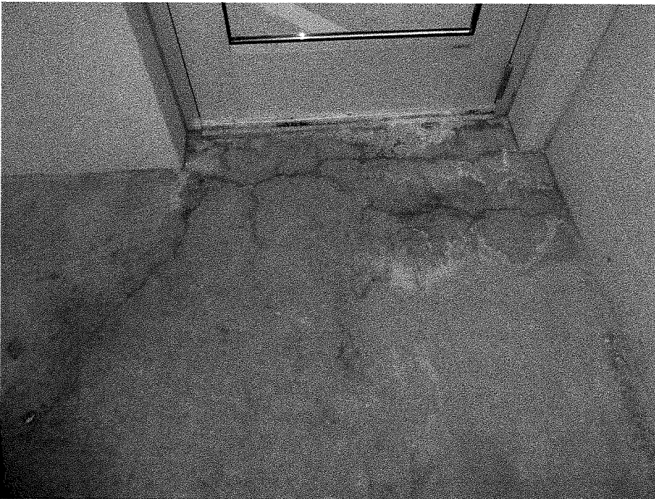
Figure 18: 6 th Street Ramp – Typical vestibule door with bristle brush sweep that allows wind-driven moisture into the vestibule.
