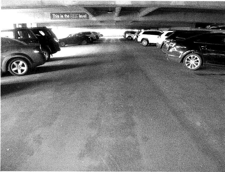
Figure 7 - Parkade Ramp – Blue Level – Old traffic coating worn away at drive lane.
