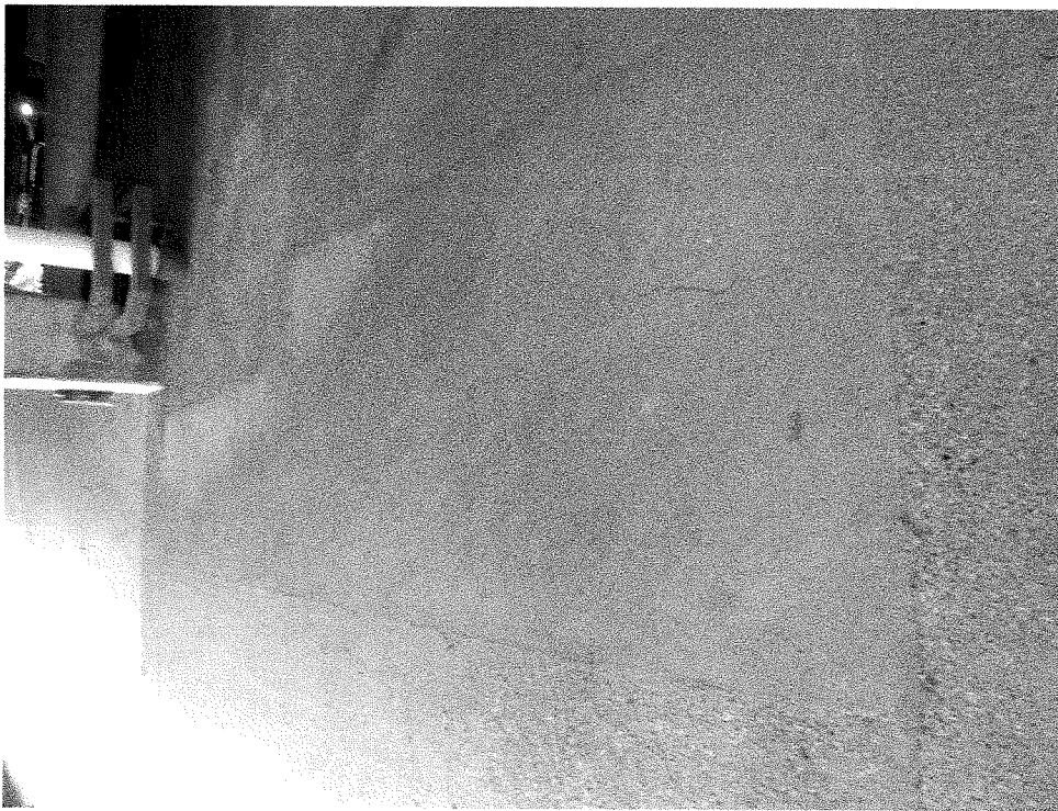
Figure 6 – Parkade Ramp – Yellow to Blue Transition – Recently patched concrete, within past year or two with shrinkage cracks that have been routed & caulked.
