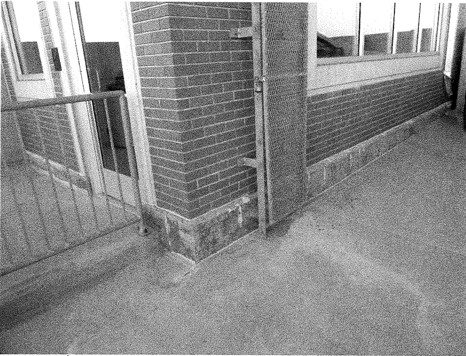
Figure 17: 6 th Street Ramp – SW stair tower at roof. Signs of moisture and concrete corrosion at base of concrete wall panel.
