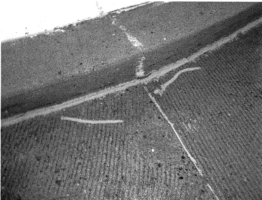
Figure 14 : Parkade – Typical caulking at inner curb of exit spiral at original slab construction joint.
