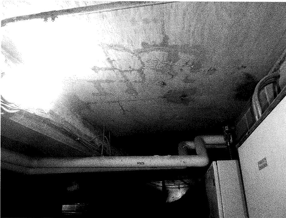
Figure 4: Parkade Ramp – Previous concrete repair patch in air handler room (below ramp entrance) showing cracking & moisture infiltration.
