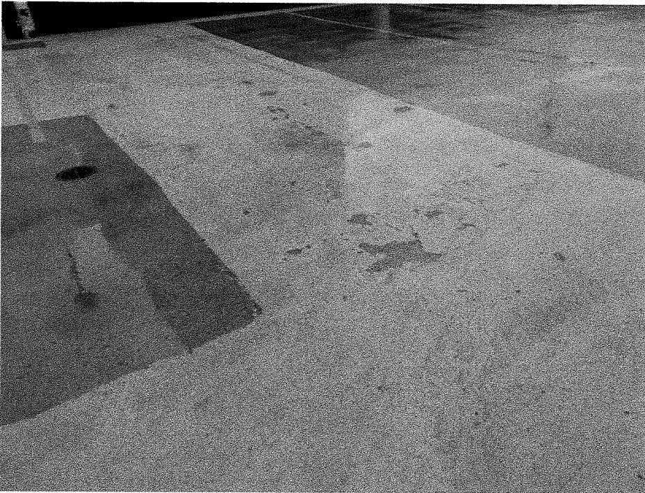
Figure 15: Galleria – Damage at existing traffic coating protecting recent repairs.
